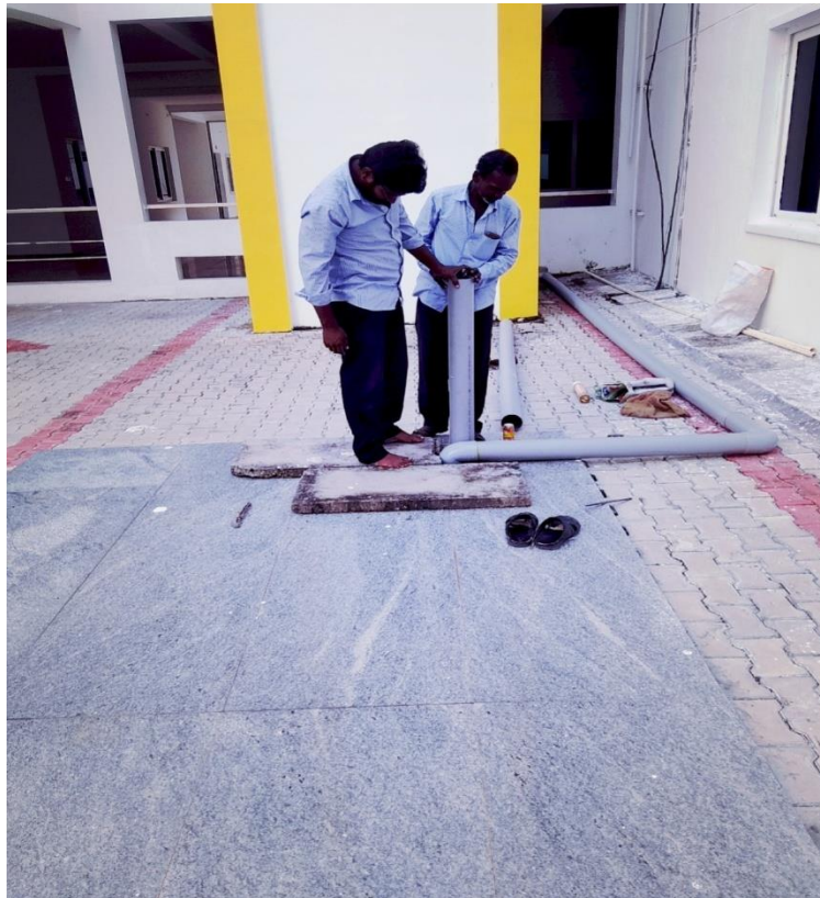
Installation works of Rain Water Harvesting Recharge Tank (20'x 8' x 15') at Engineering Block
