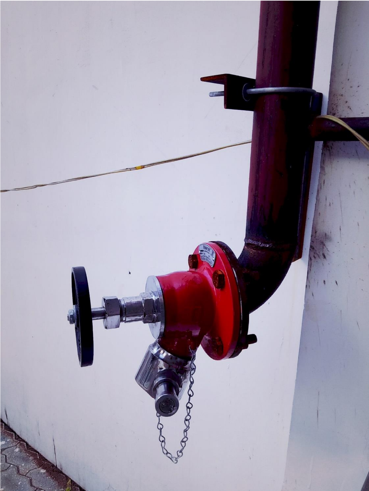
Fire Hydrant at Main Block
