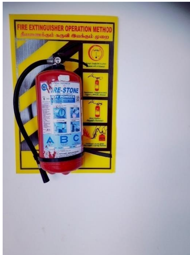
Fire Extinguisher at Engineering Block
