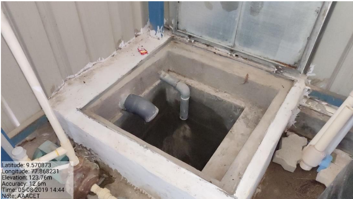
Rain Water Harvesting Tank
