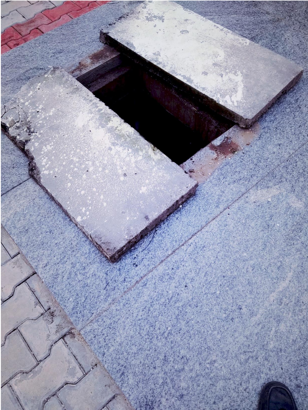
Rain water harvesting Recharge Well at Engineering Block
